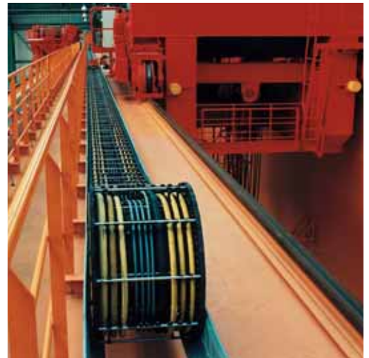
318 for long travel distance on a crane application.
